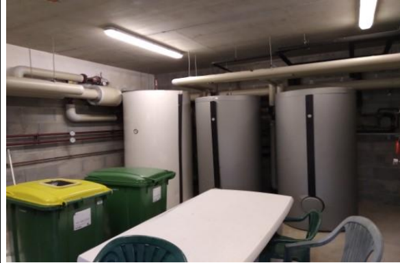
Ballons de stockage ECS
